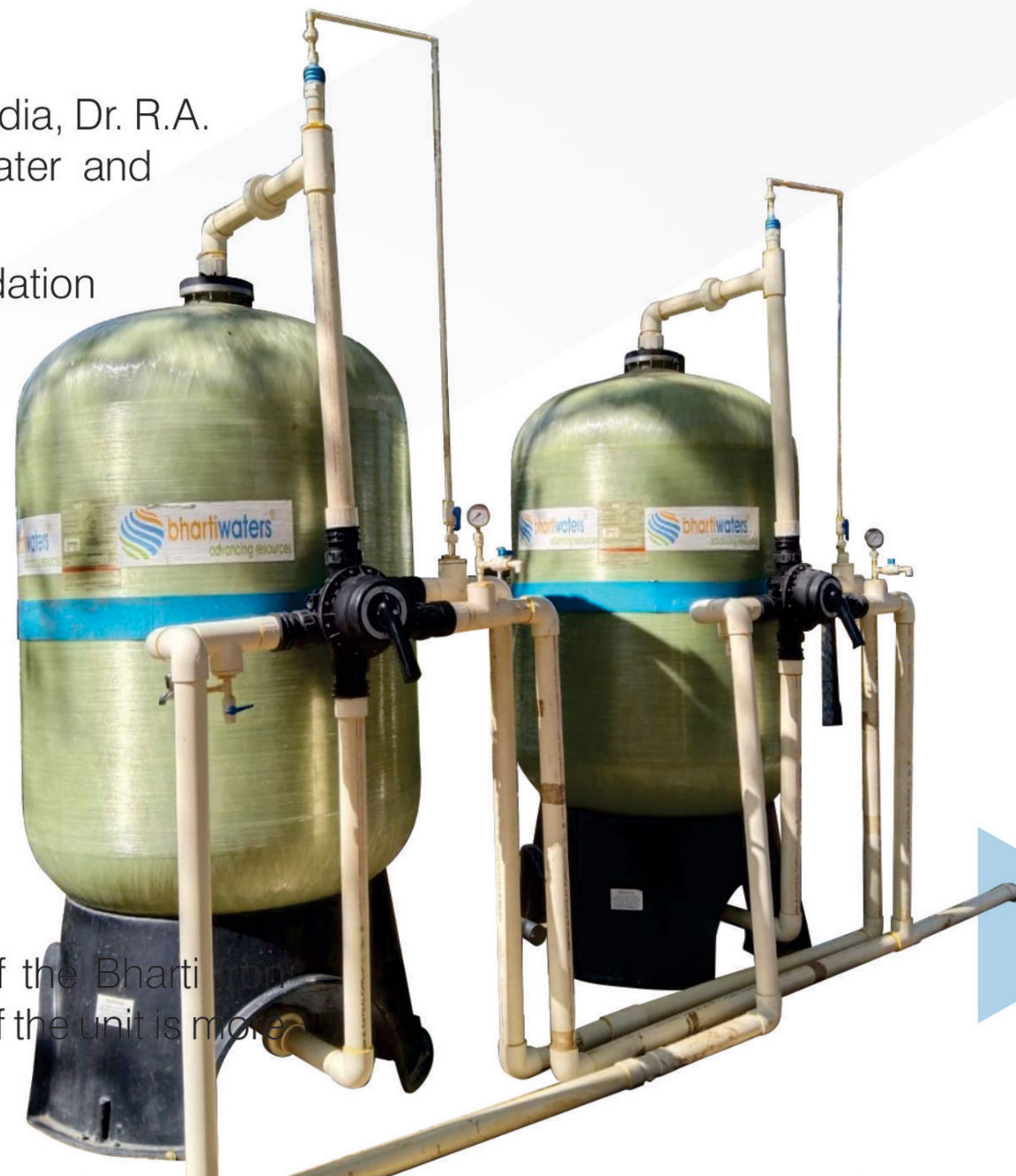
69m 3 /hr plant installed in MES Dinjan, Assam
